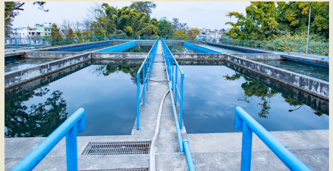
Bansbari Water Treatment Plant
