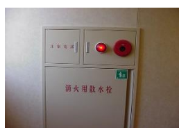
Left: Emergency Telephone Right: Alarm Button Bottom: Fire Hose
